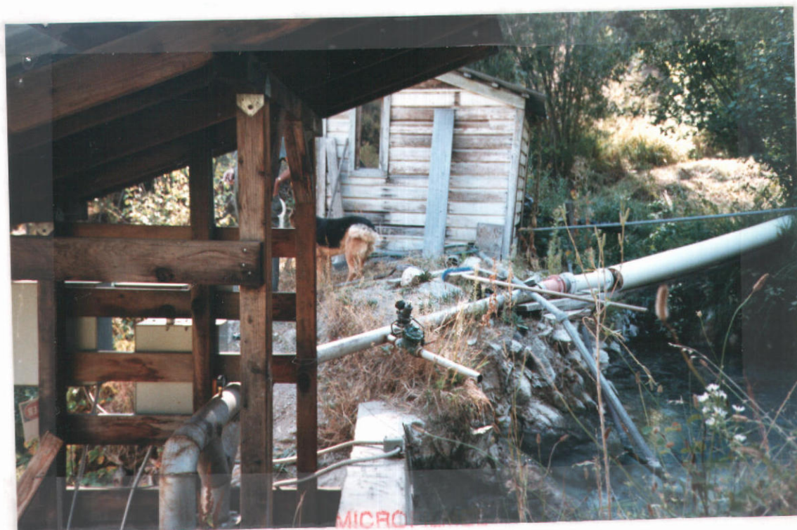
Pipes Leading up hill TO HOMES
