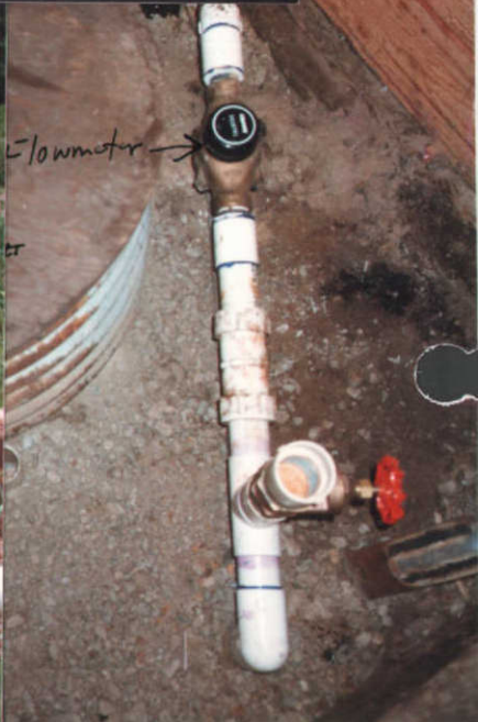
⑤ Mainline from well #2 emerges in bottom of photo and is reburied in top of photo. Note flow- meter in middle.
