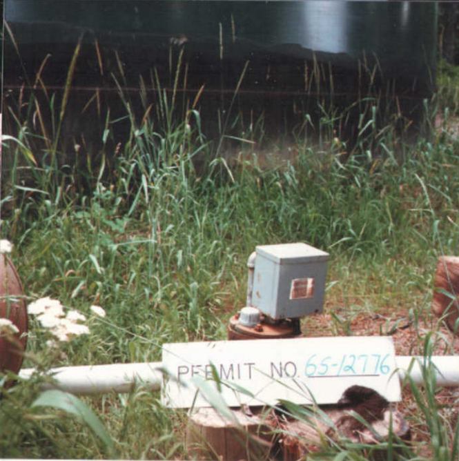
④ P/D #2 Well in foreground and 40,000 gallon tank in background.
