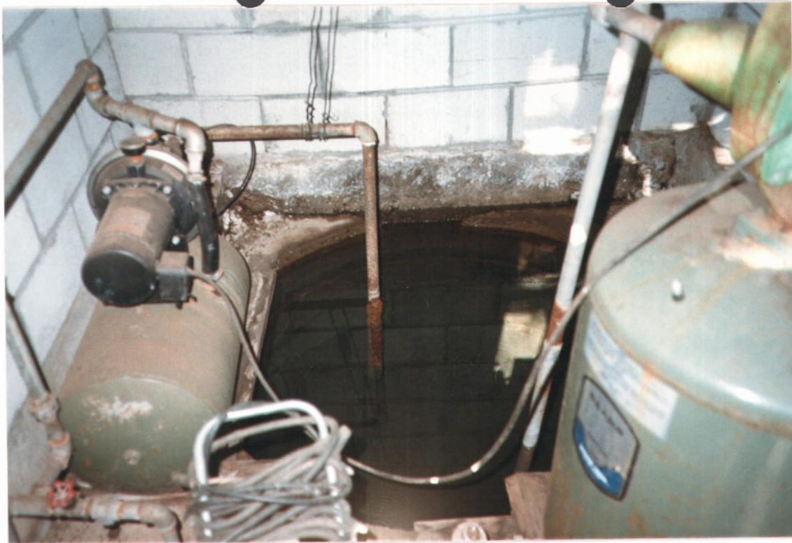
Pump house set-up
