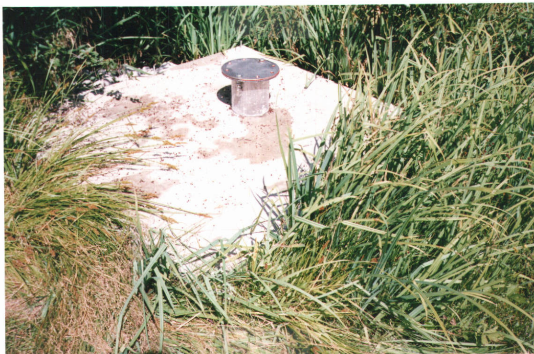
PHOTO ONE- An 10" diameter stand pipe and 6" concrete cover over 22' deep spring development.
