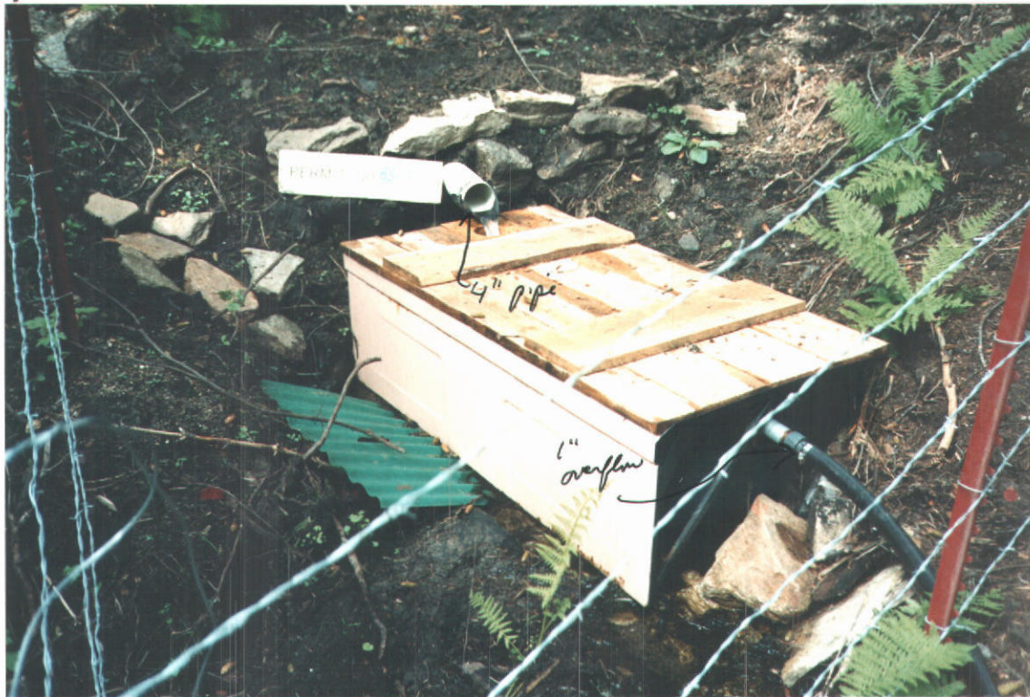
PHOTO ONE- P/O - spring box (buried) with 4" pipe to tank, 1" overflow to stream. can use portable pump at tank.
