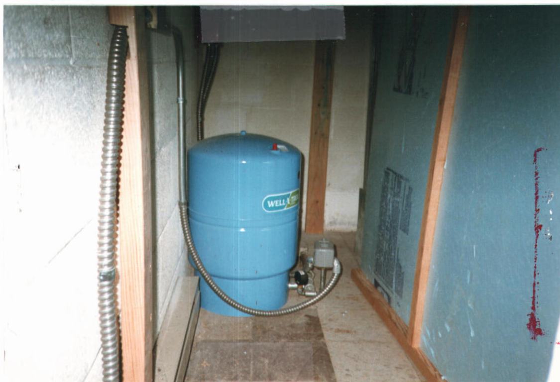
PRESSURE TANK IN STORAGE BUILDING
