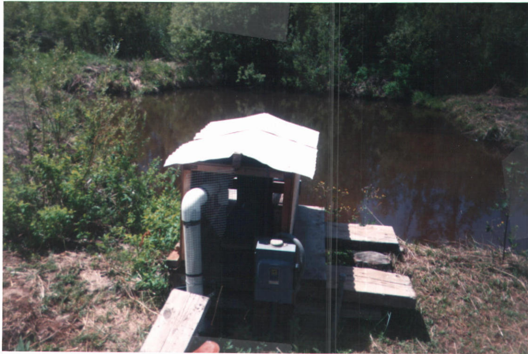
Pump #2 and pond #2.
