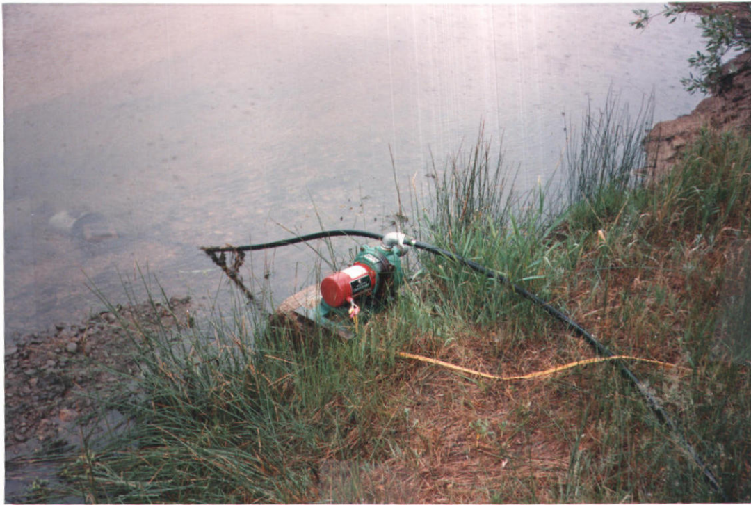
Pump located on bank of Puyette River, N. Fork 1" discharge.
