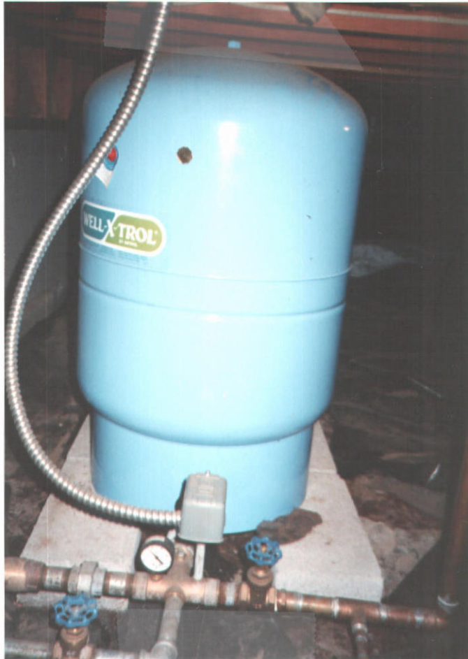
#1 Pressure tank inside house.
