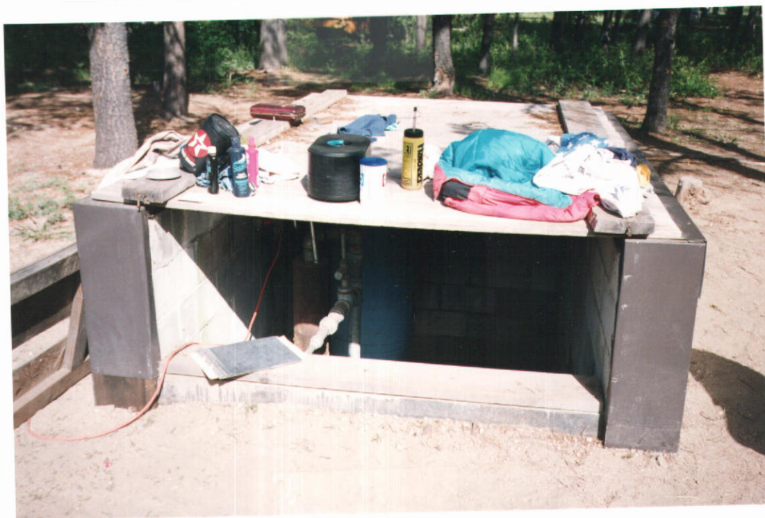
PHOTO ONE- Well and pump house located in center of compound.
