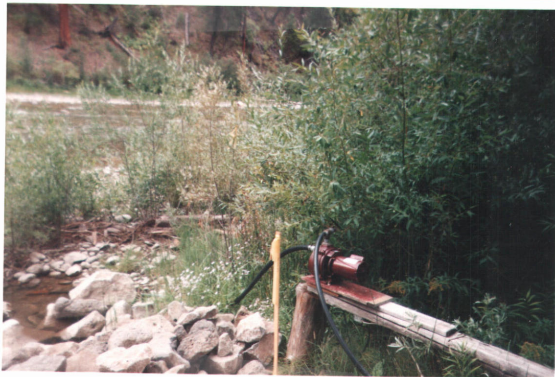
View of pump on S. Fork of the payette, @ South of Propuley.
