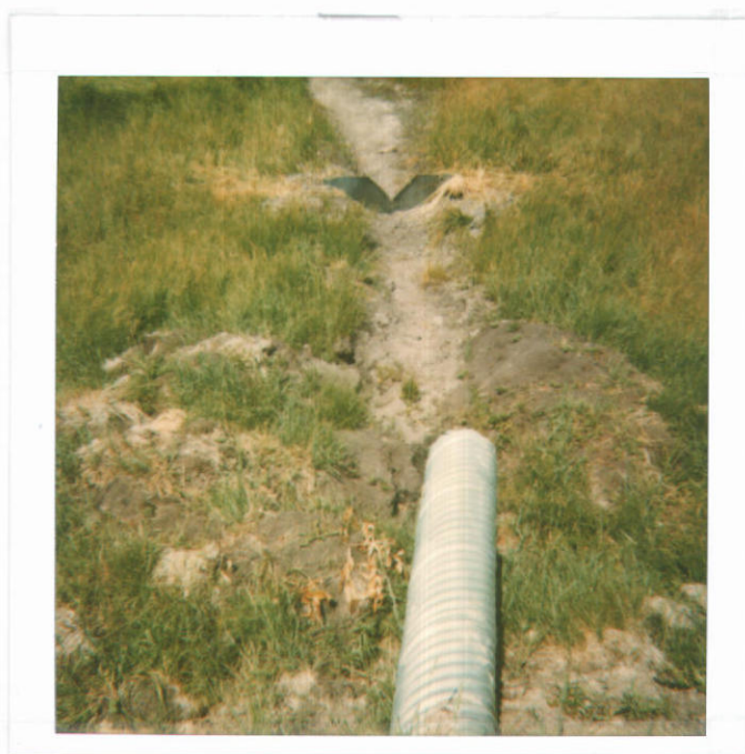
Outlet and Downstream V Notch
