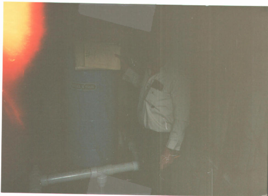
#1 a poor picture of the inside of pump house #1
