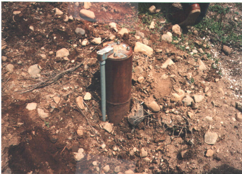
#2 6" casing for well #1 located adjacent to pump house #1
