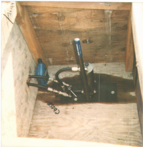
TOM J DAM OUTLET GATE CONTROL 65-13019 4/26/96
