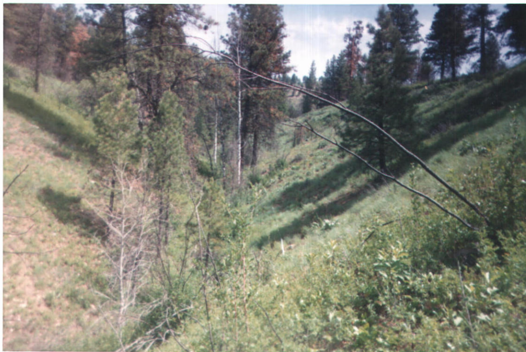
2" PVC extending up Ravine to springs. View to the NW.
