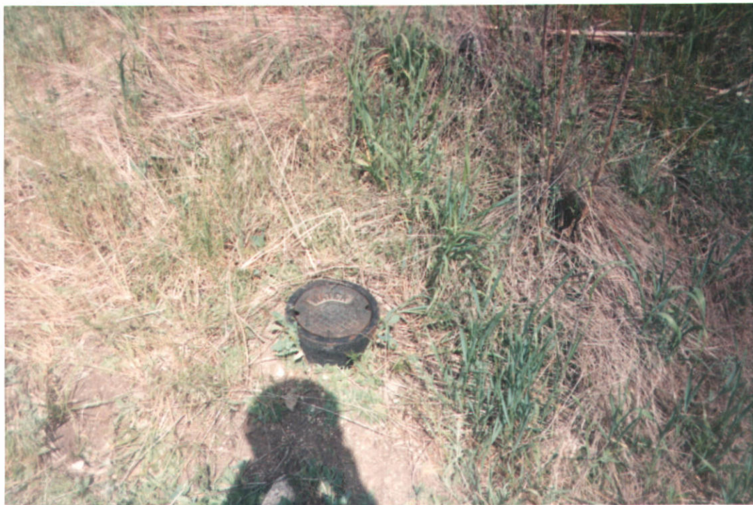
Valve NW of pumphouse. A 2\frac{1}{2} " line from pumphouse and a 4" line to subdivision intersect at this valve.
