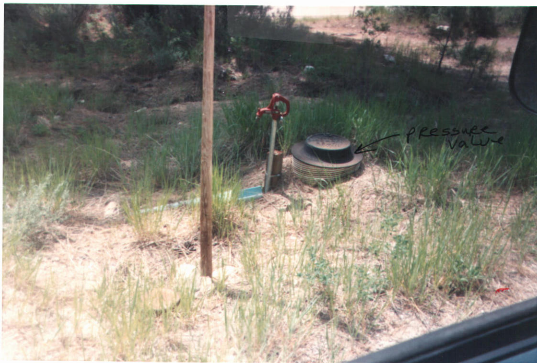
Pressure valve and 1 of 2 4" valves located between Aspen Way and Hwy. This 4" valve supplies water under Hwy to Scenic Properties Sub. No. 1 & 3 located south of Hwy.
