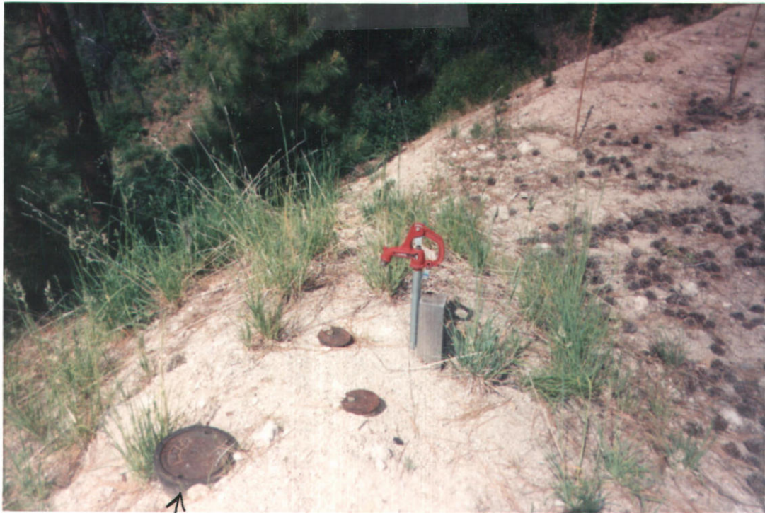
Water Valve for 4" Line to subdivision. Two Valves for 4" overflow.
