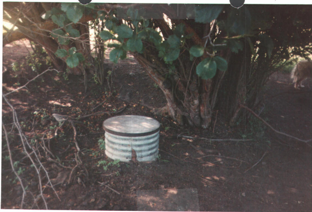
2' diameter CMP STAND pipe in spring. Water is piped by gravity through 1½" PVC to water Trough approx. 150' to the west.
