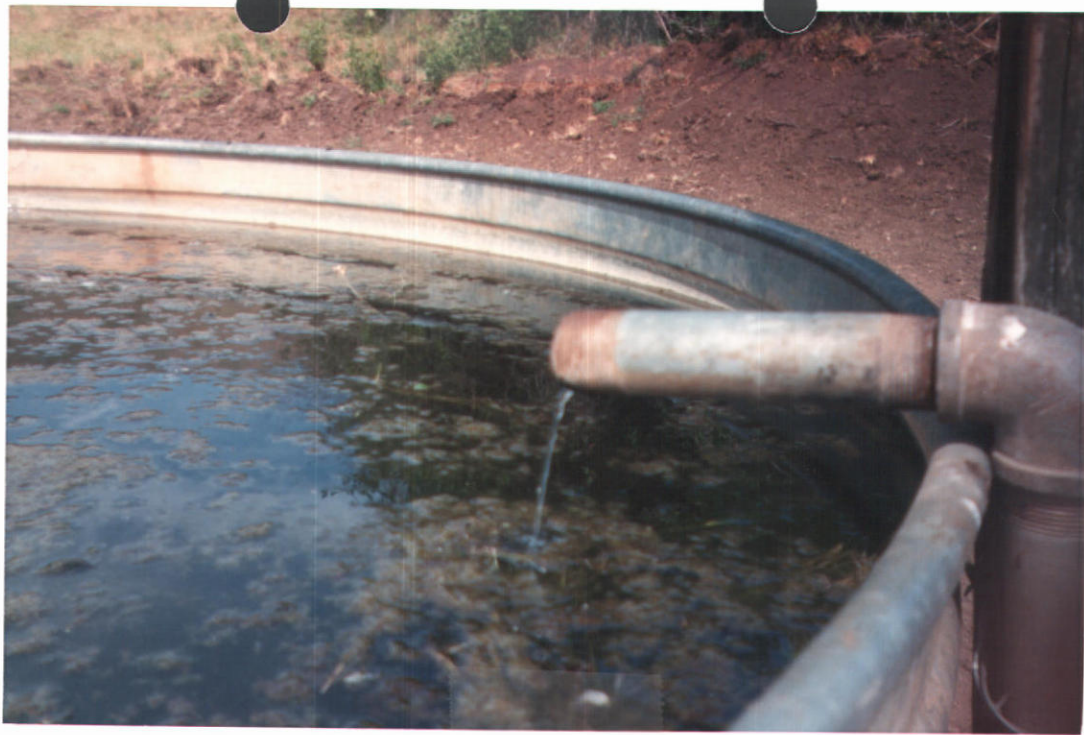
Flow into water Trough.
