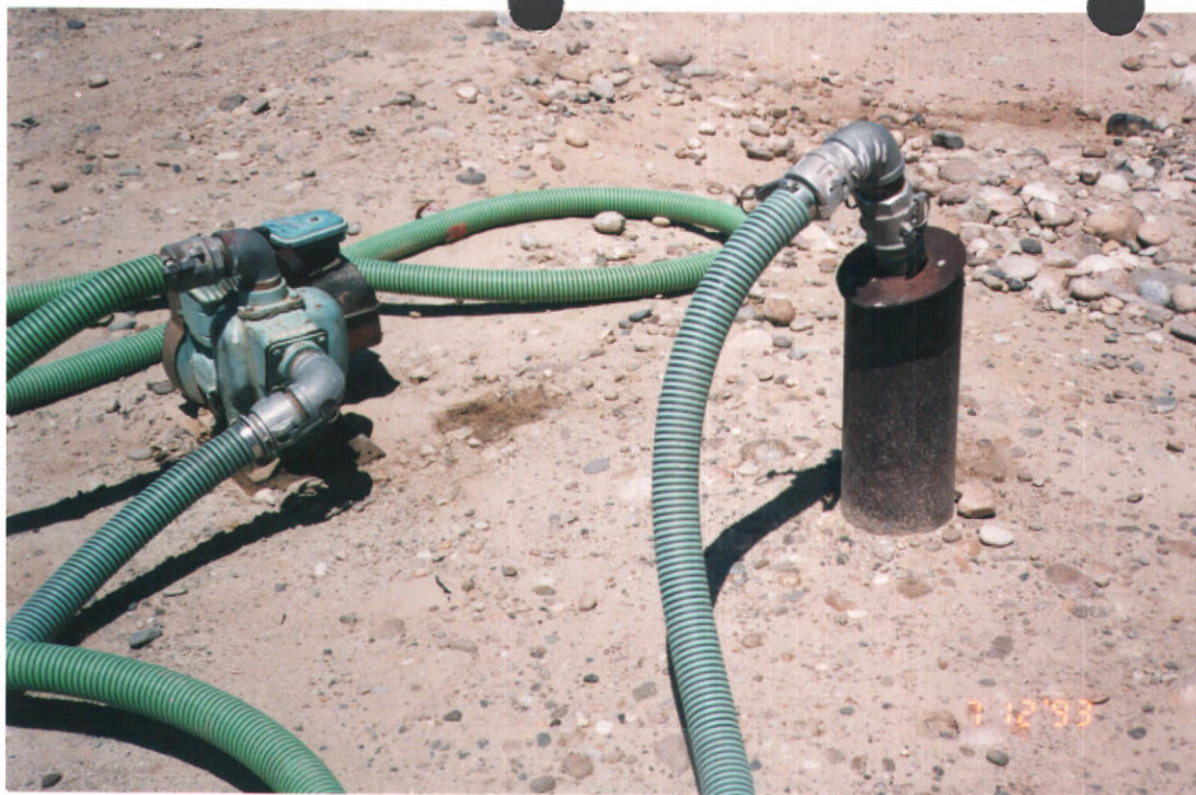
Well #1 (West well) 5HP portable pump
