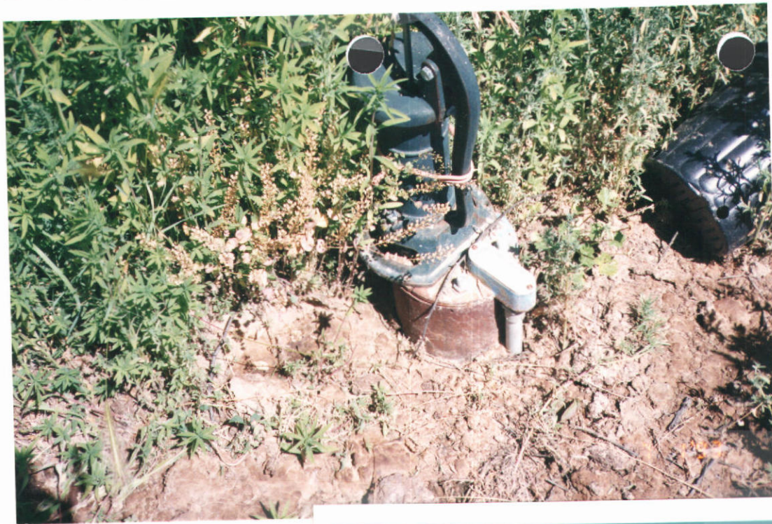
6" well 1 hp submersible pump (hand pump on top)
