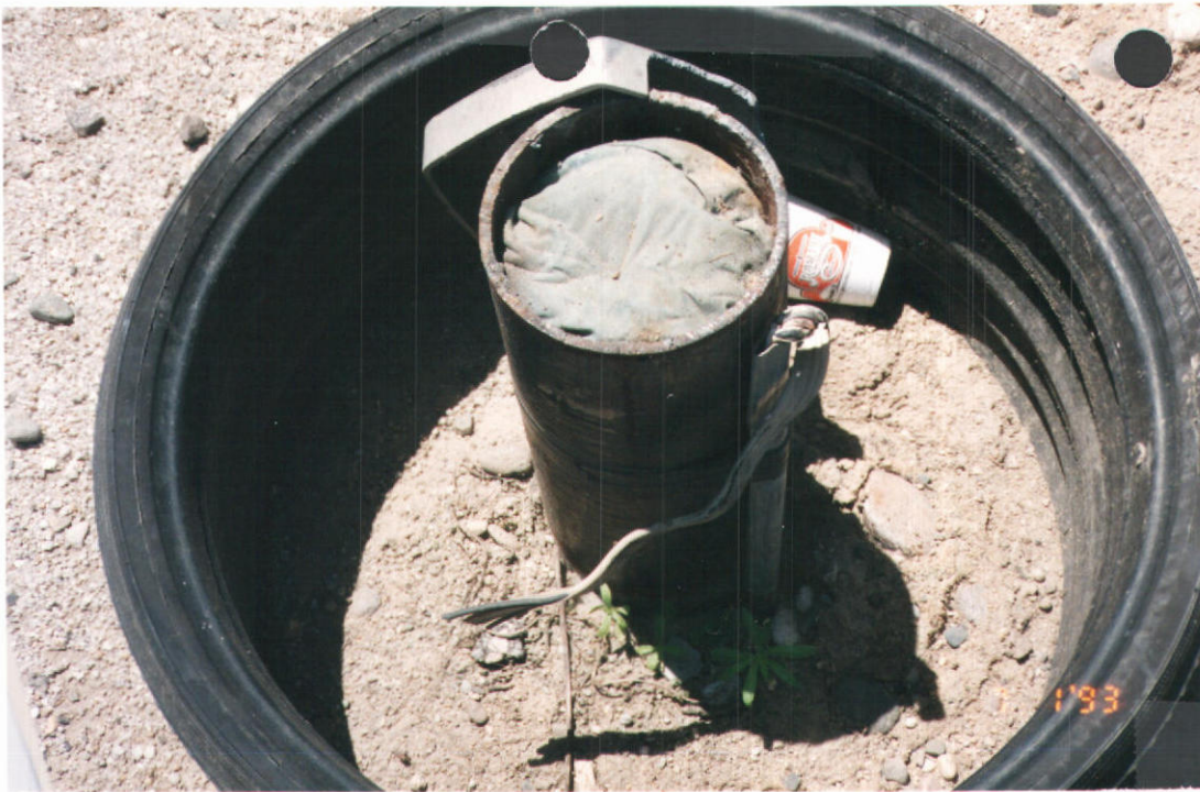
6" well 1/2 HP submersible pump
