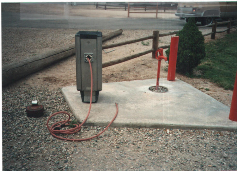
#1 Point of diversion and one outside faucet.
