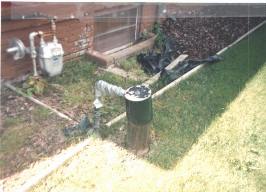
#2 view of the well. Notice the line submerging underground. Location on the north side of building.
