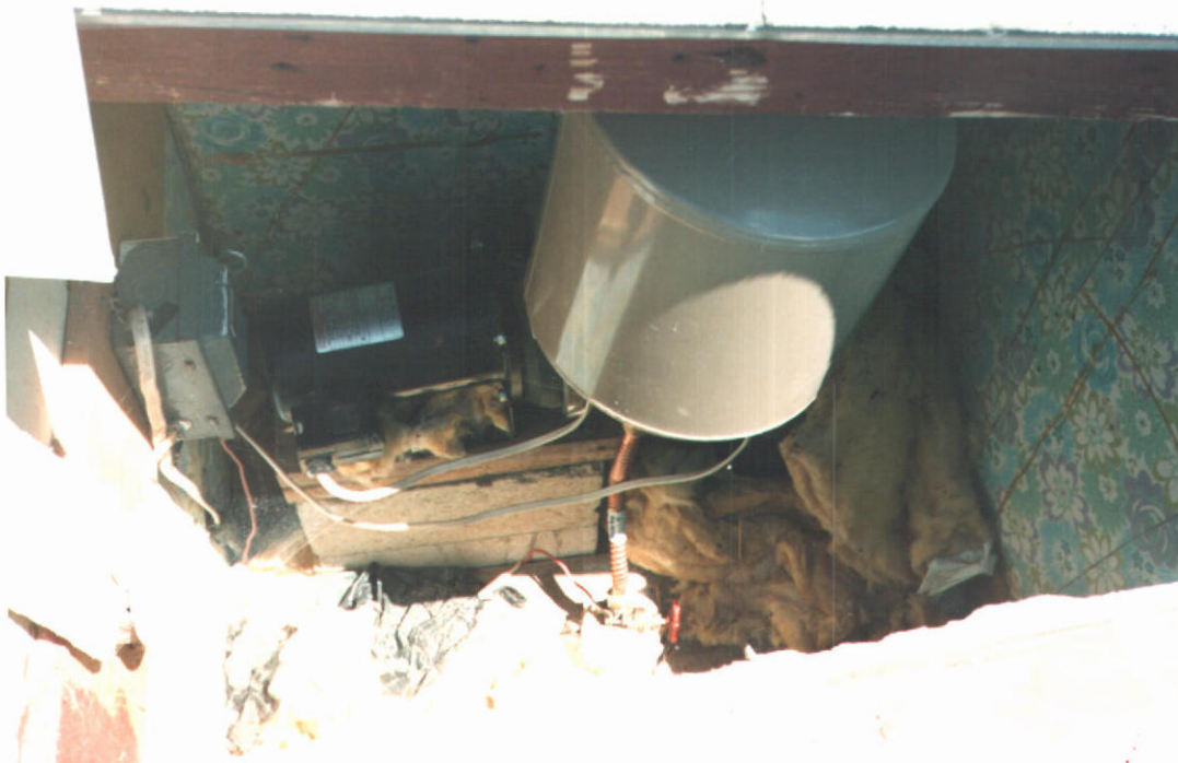
#2 View looking inside wellhouse
