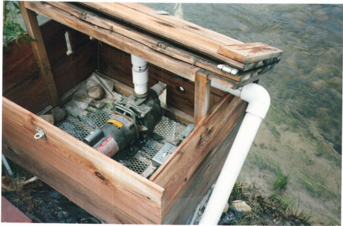
PHOTO ONE- Pump and motor in enclosed structure at edge of river.
