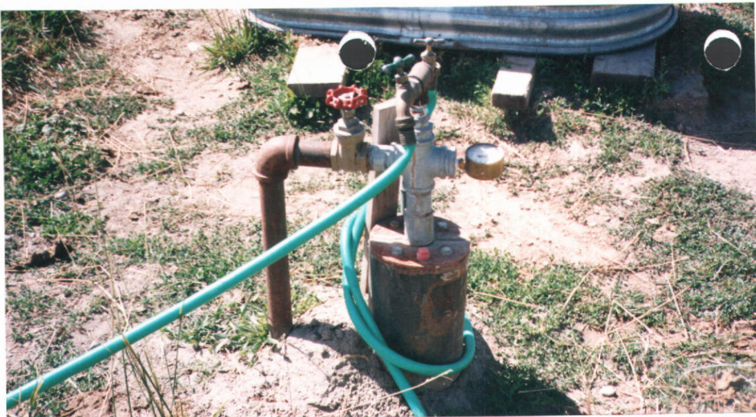
6" well 1 HP submersible pump
