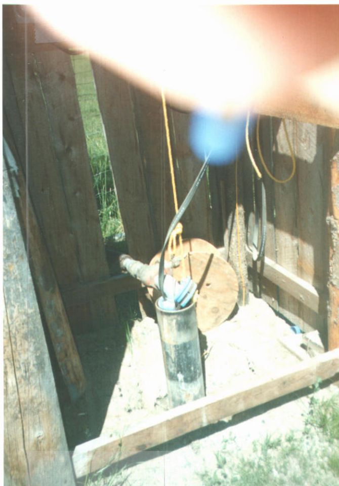
WELL AND LINE HEADING TO LOWER MAIN- LINE OF THE PROPERTY.
