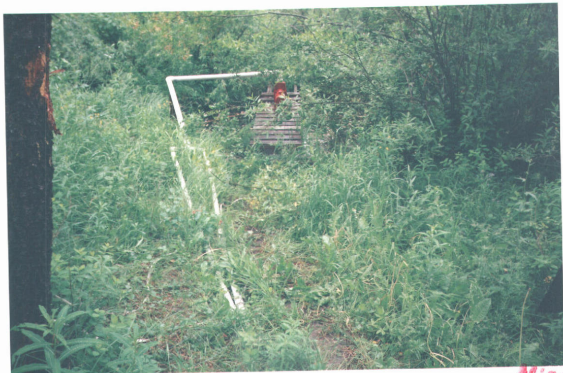
PHOTO TWO- Pump and distribution system to underground sprinkling system.
