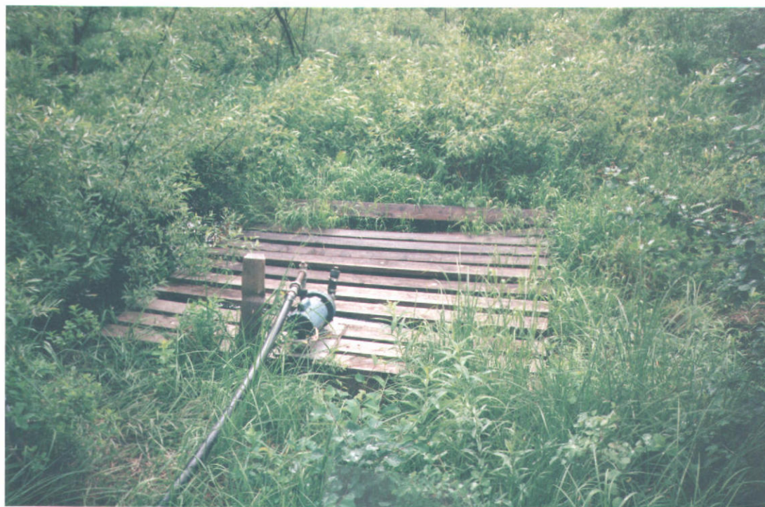
PHOTO ONE- Pump mounted on boards over dugout spring depression.
