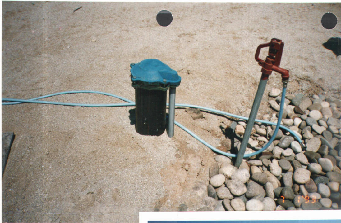
6" well 1/2 HP submersible pump
