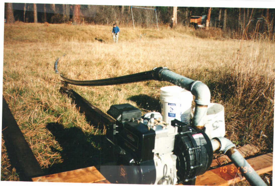
1 1/2" discharge Flood Irrig
