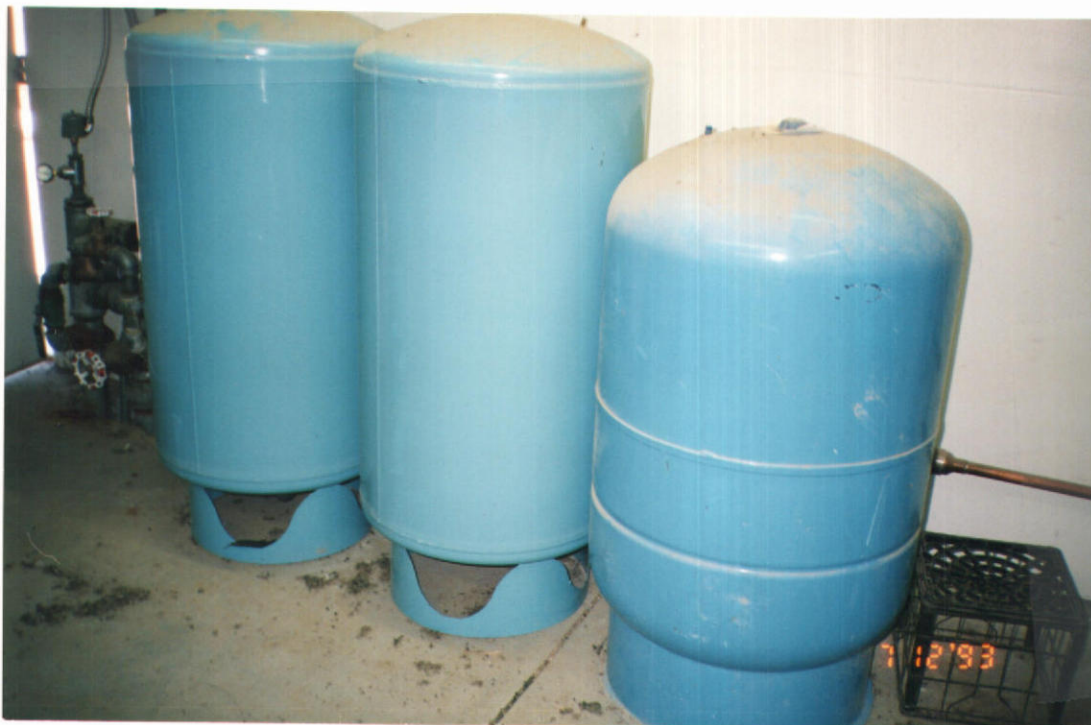
Three 150 gal storage tanks
