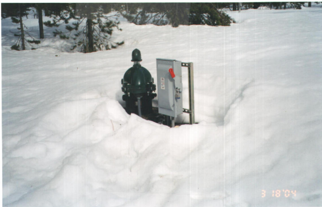
10" WELL #2 25 HP SUB. PUMP
