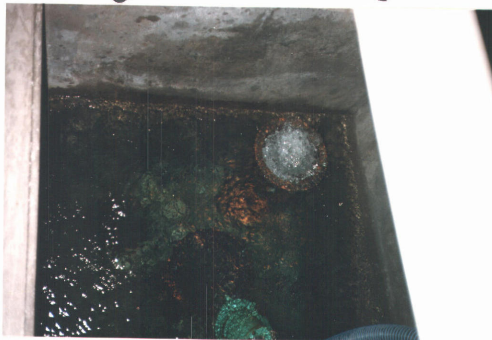
Looking Inside Control Box
