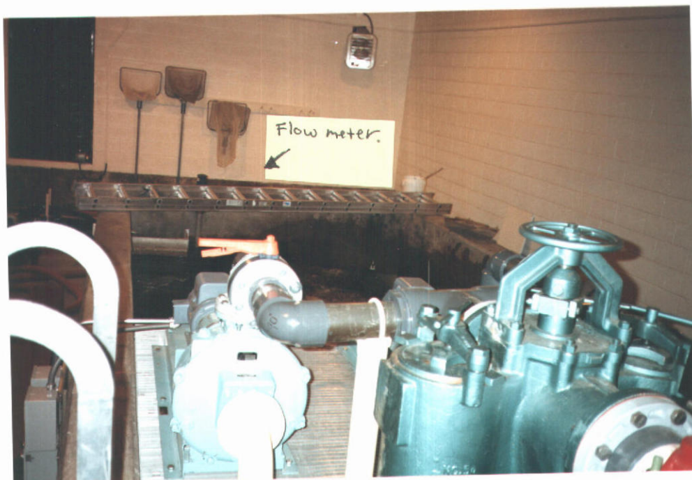
Head Box inside Control Box inside Hatchery Building where Water is diverted to different uses in Hatchery.
