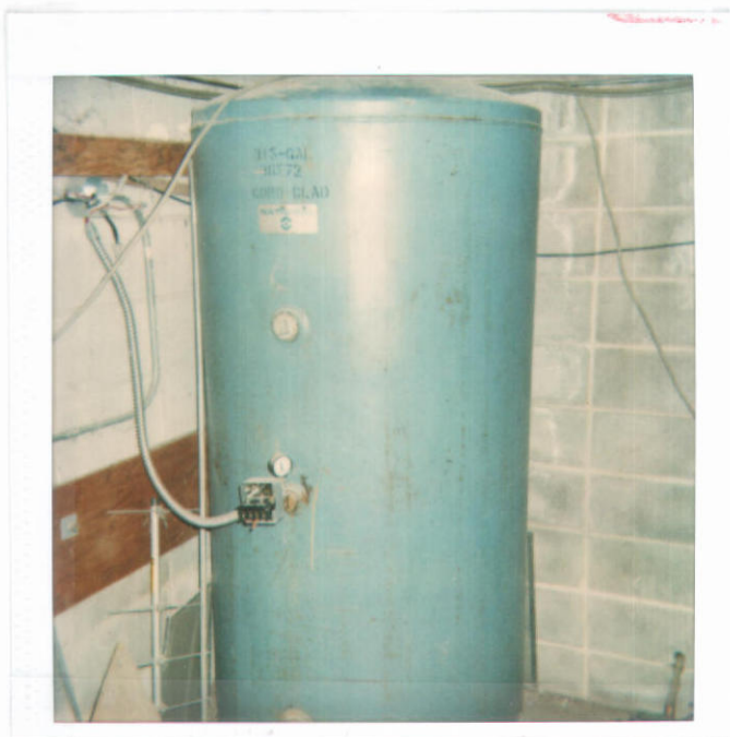
Pressure Tank - Motel
