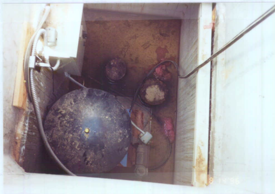
This is well # 17. This well is connected TO THE main line FROM Pump 19 BUT IS NOT ASSOCIATED WITH THIS PERMIT.
