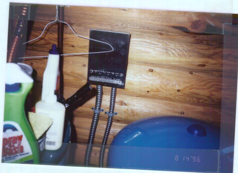
This is the pump control box inside the house.
