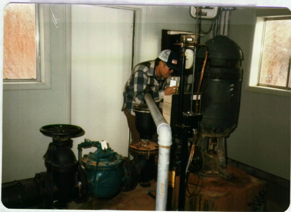
Pumphouse Interior West Well #1
