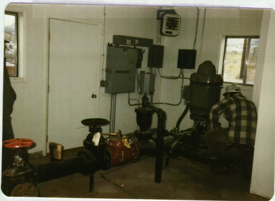
Pumphouse Interior East Well
