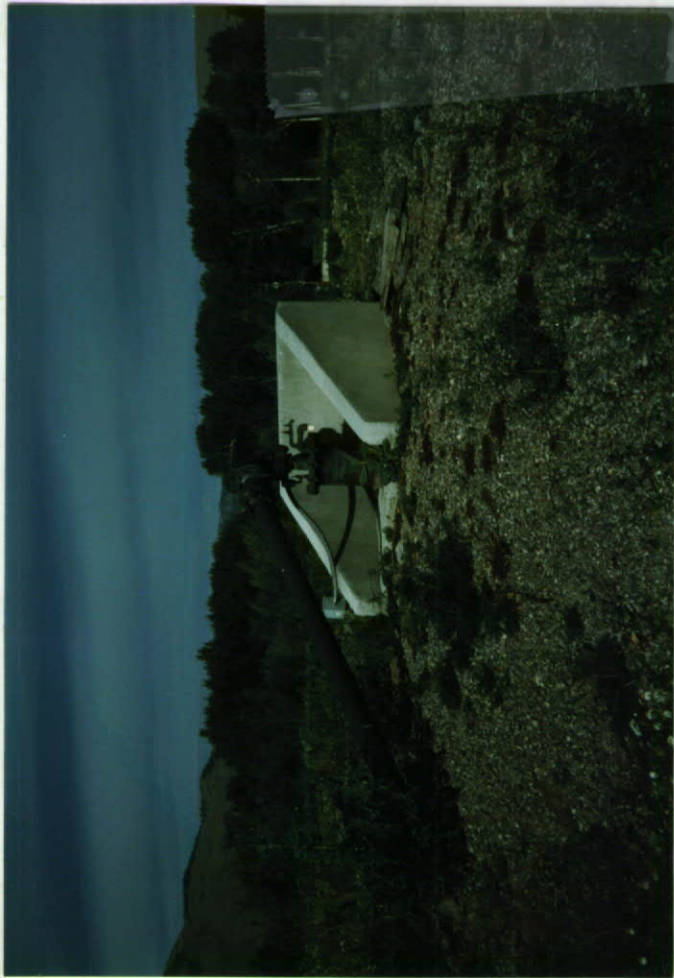
WELL WITH SUBMERSIBLE MOTOR AND PUMP.
