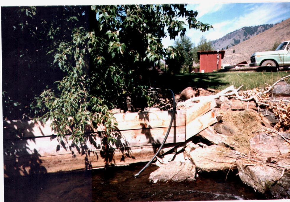
Intake in Thompson Creek, PU in Background
