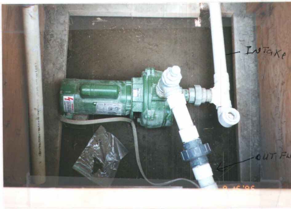
2 HP Pump FOR PID OUT OF SALMON RIVER
