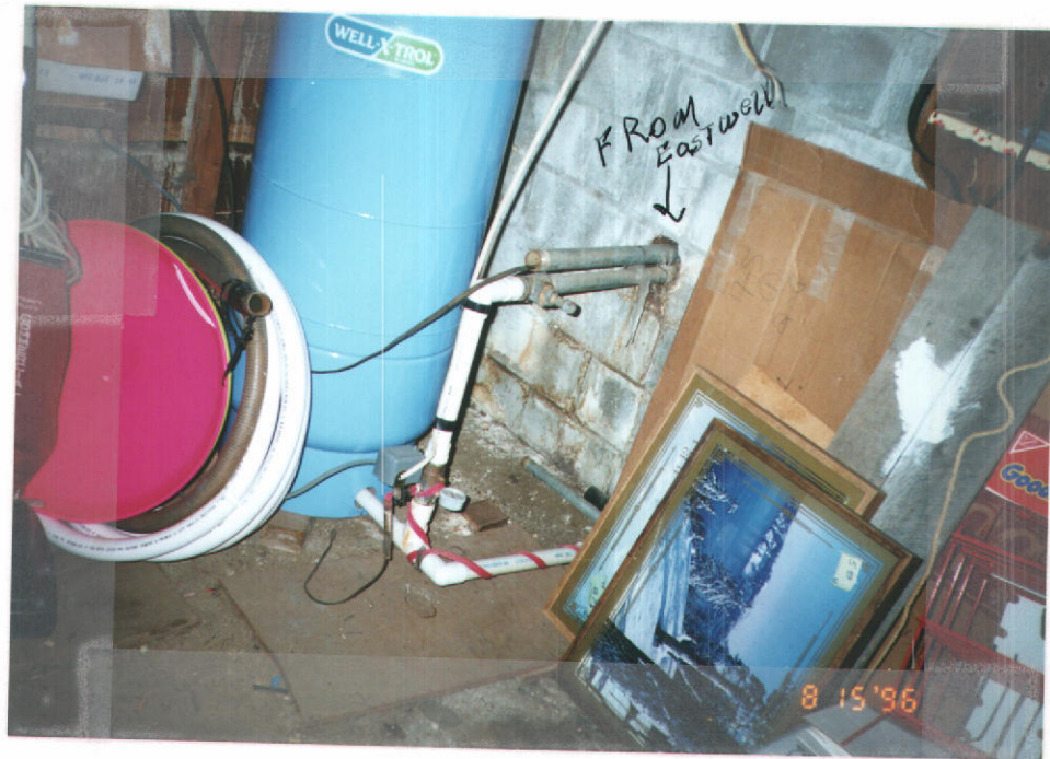
EAST well ENTERS Lodge HERE and ENTERS PRESSURE TANK.
