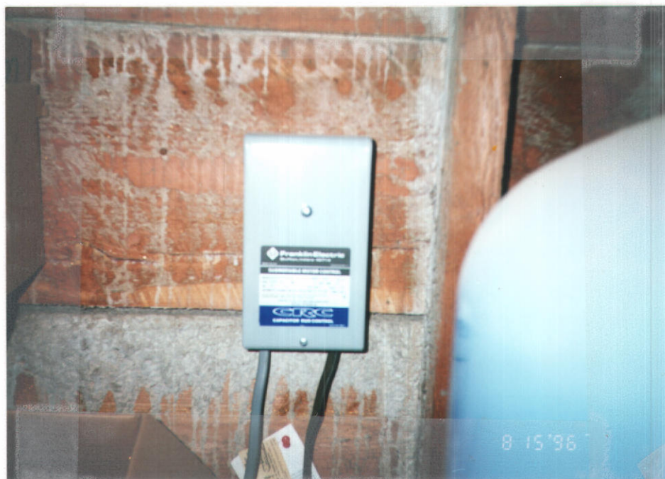
CONTROL BOX FOR EAST well.
