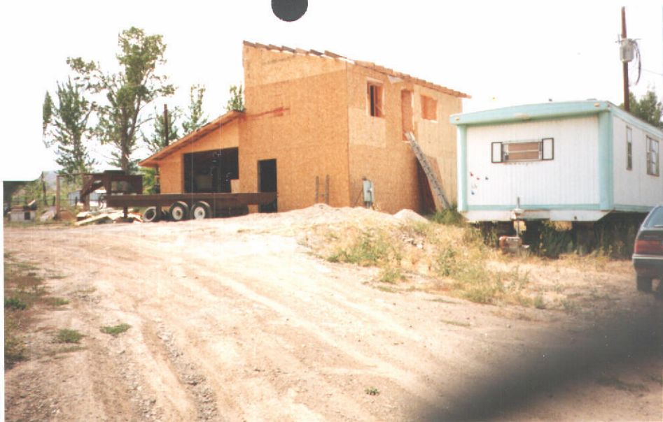
72-07502 HOUSE/SHOP UNDER CONSTRUCTION PLUMBING CONNECTED TO WELL
