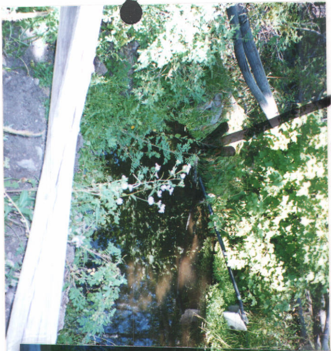
Diversion Pipeline to Guervo sprinklers
