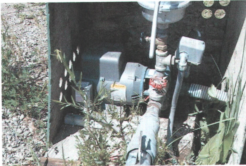
Permit 72-7564 POD. Baldor 5 HP motor 8-14-03
