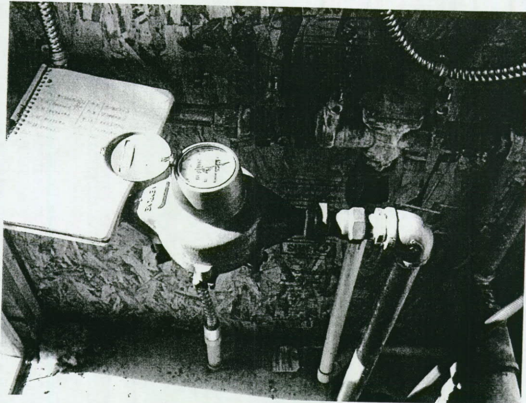
Photo 2. Well #2 flowmeter and connection piping to potable water system.
