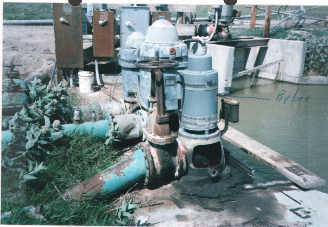
- 40 HP Pump at Bybee Reservoir -
