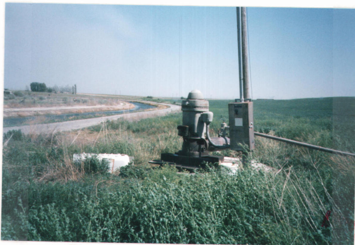
- 100 HP Booster Pump From Canal -
