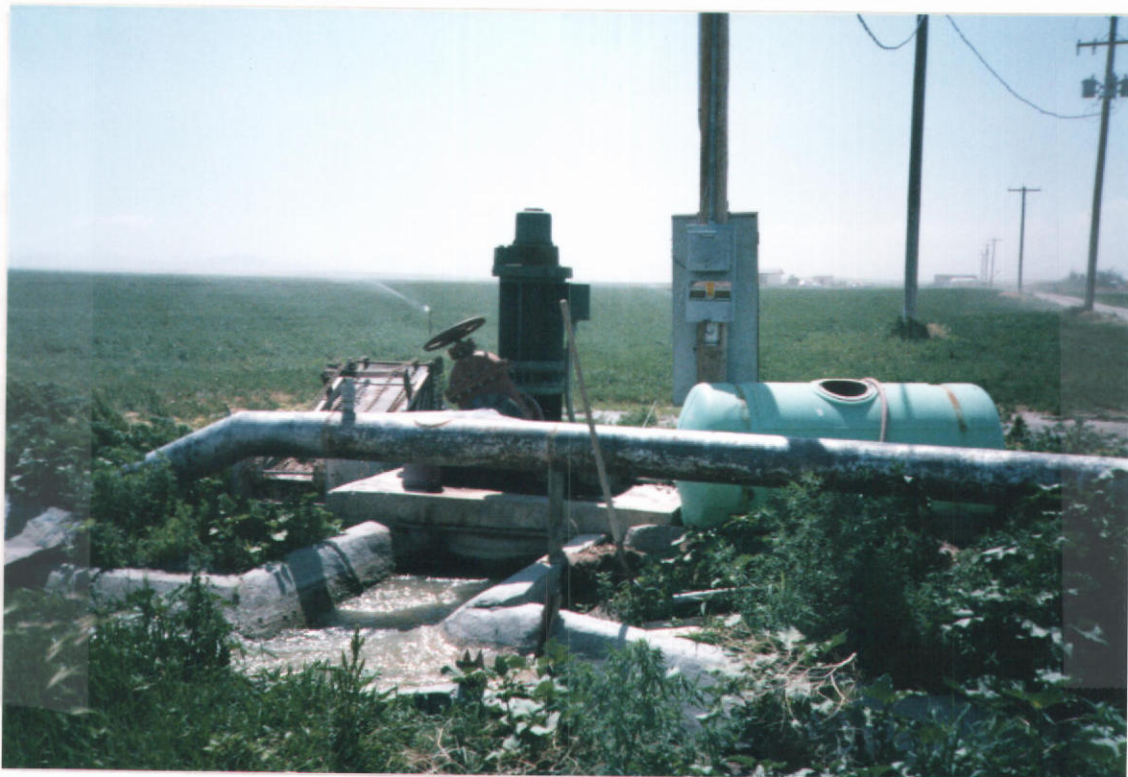
- Bybee Relift Pump - 100 HP -
