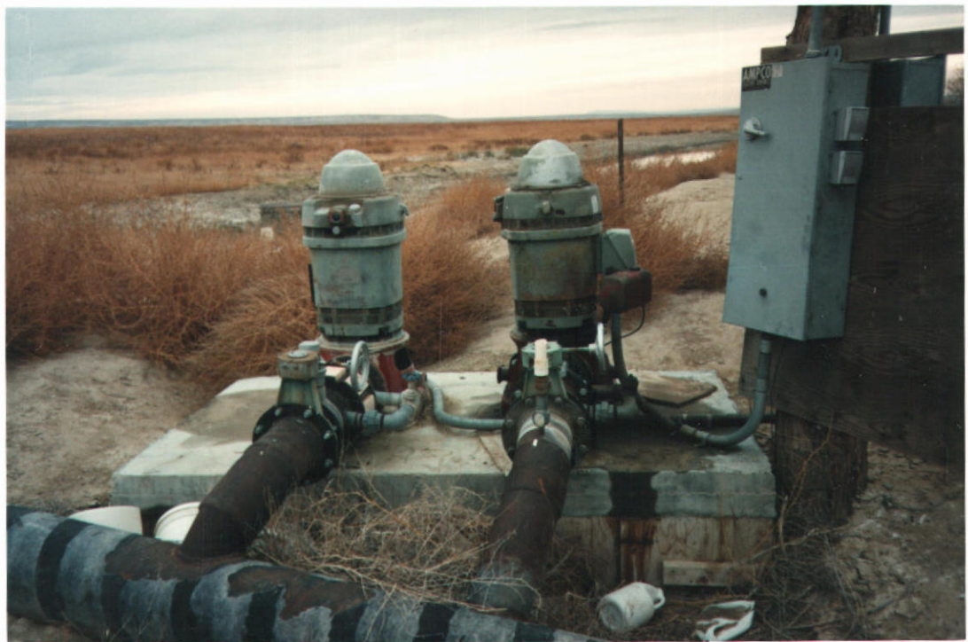
TWIN LIFT PUMPS
