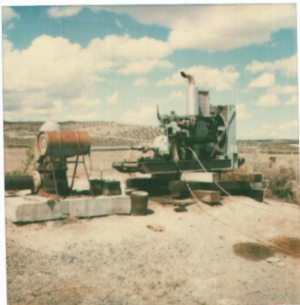
ROCK HOUSE RANCH PUMP # 2
