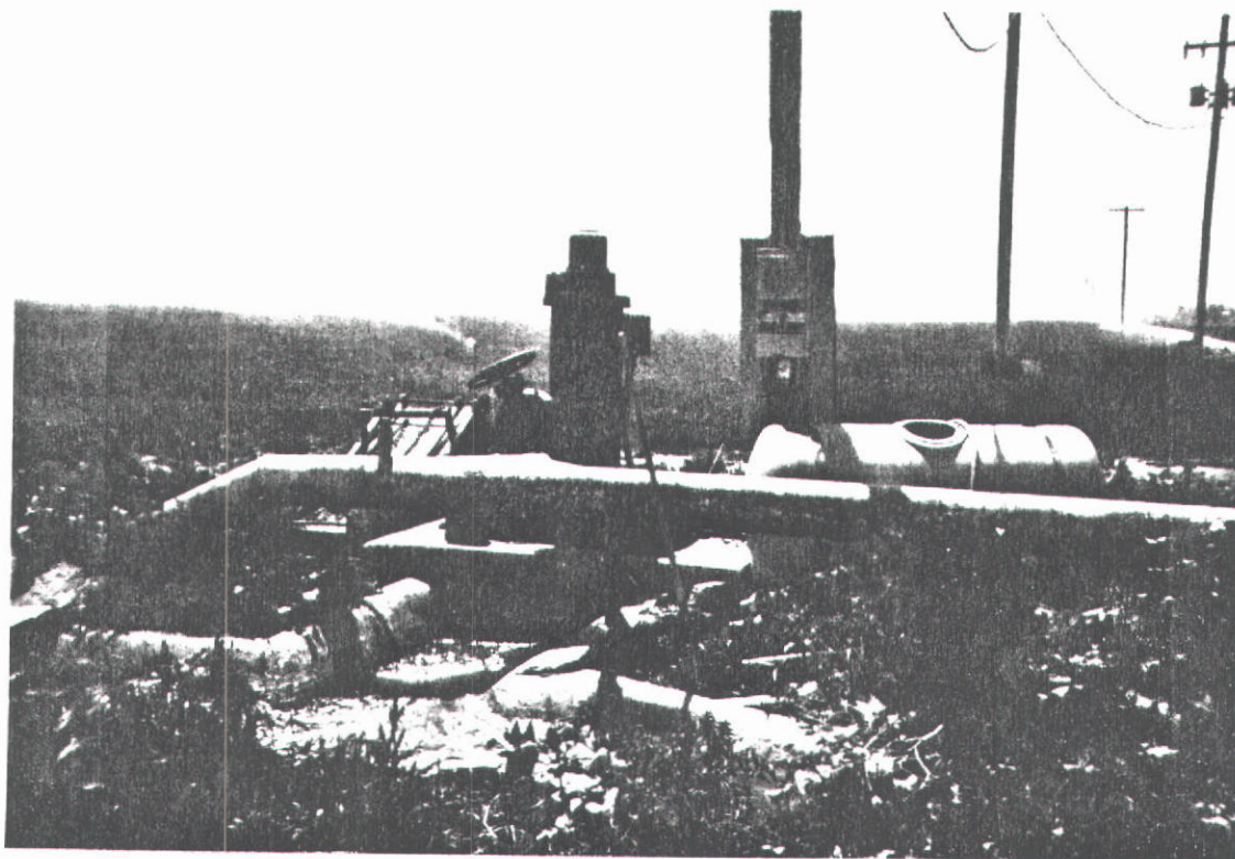
- Bybee Relift Pump - 100 HP -
