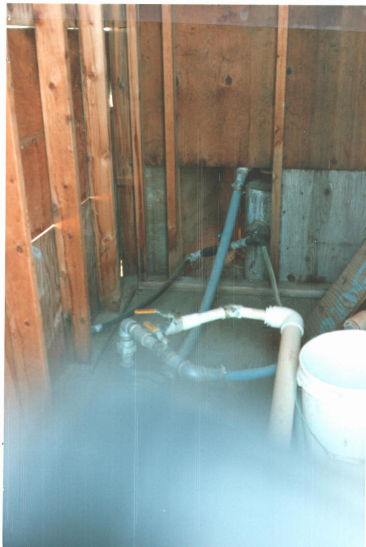
PICTURE # 2. SHOWS INSIDE OF WELL HOUSE.
